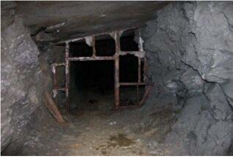
Remains of a doorway used to control air circulation in the mine
